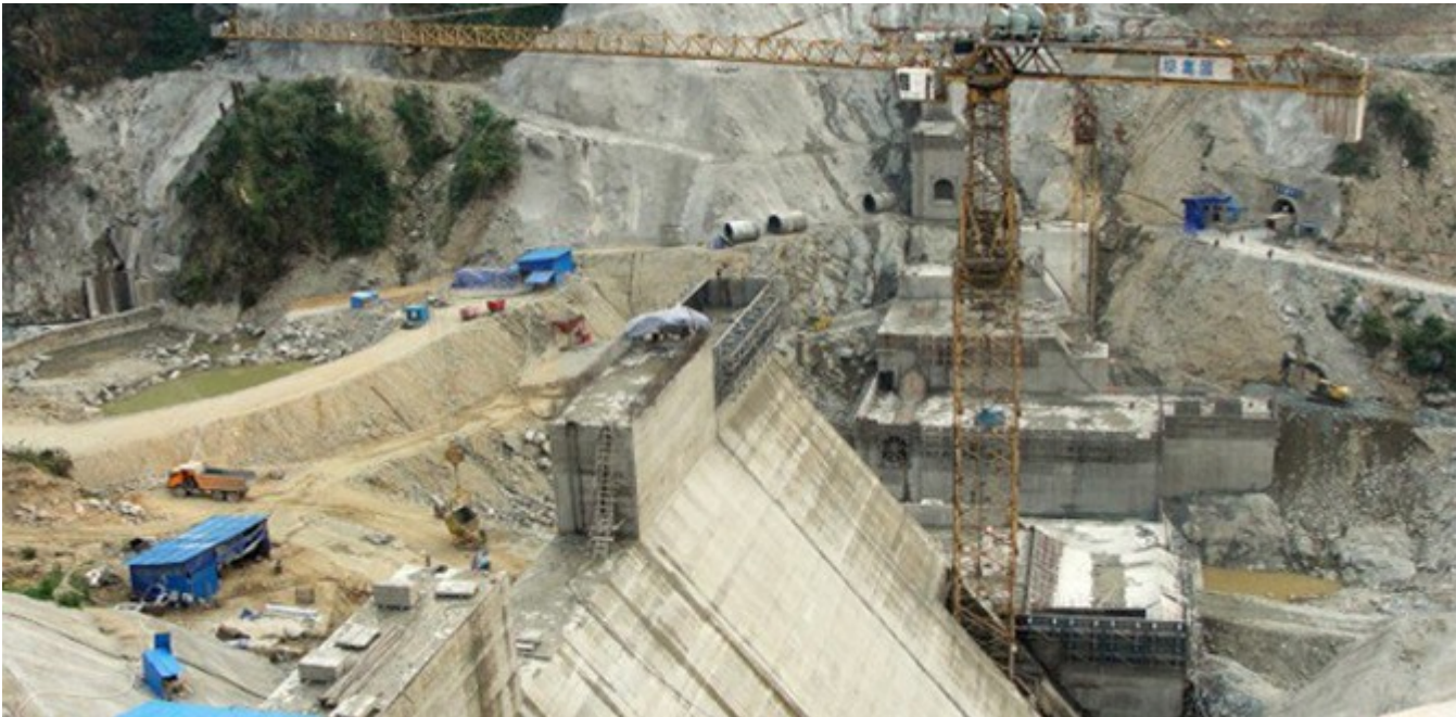
Construction at the Myitsone Dam, a megadam project on the Irrawaddy River. (PHOTO: Jingpaw Targyi)
